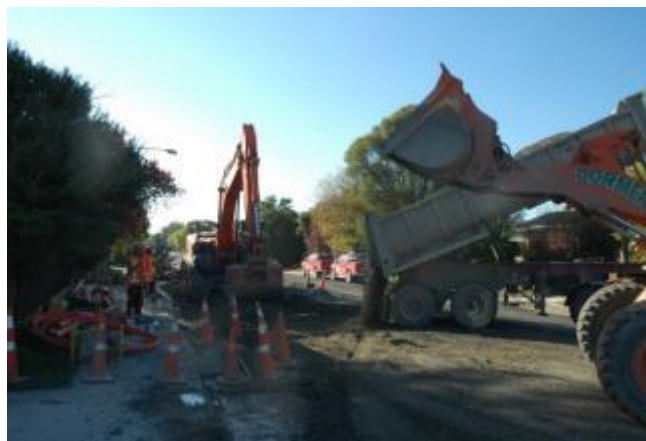
Photo 8.43: Excavation and backfilling due to use of open-cut method in very loose soil (Sep 2010 Kaiapoi) (Source: Author's own)
