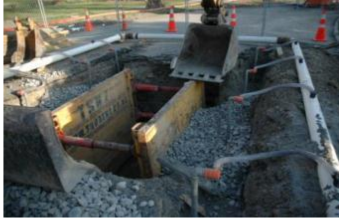
Photo 8.45: Wastewater pipe localised open-cut repair with supporting box in loose sand under water table (25 Sep. 2010, Avonside, Christchurch) (Source: Author's own)
