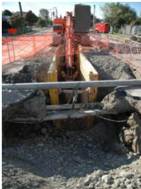
Photo 8.46: Wastewater pipe localised open-cut repair with supporting box in loose sand and dry soil (25 Sep.2010, Darlington Christchurch, Source: Author's own)
