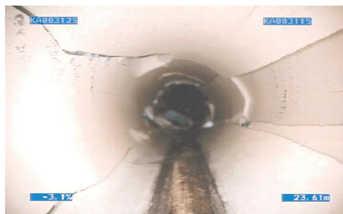
Photo 8.53: Severely damaged wastewater pipe (Source: Christchurch (Gordon, 2010))
