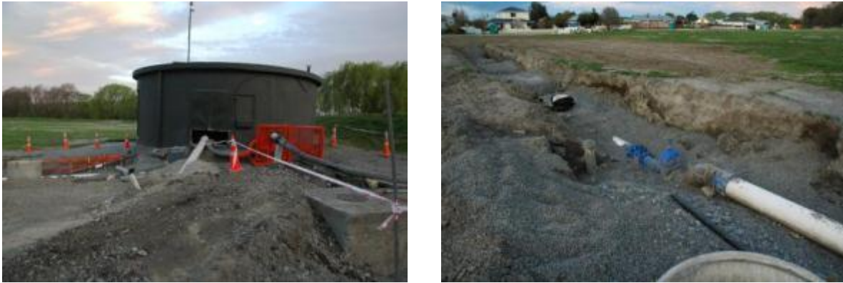
a b Figure 8.17: Main WWPS failure in Waimakariri District (Kaiapoi 24 September 2010) (Source: Author's own)
