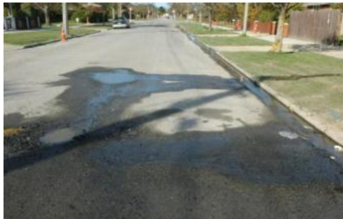
Photo 8.54: Visual inspection (water invasion) (Source: Author's own)
