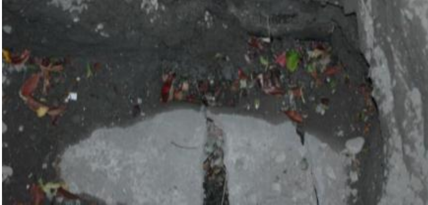
Photo 8.24: Main sewer breakages in Avonside, 25 September 2010 (Source: Author's own)
