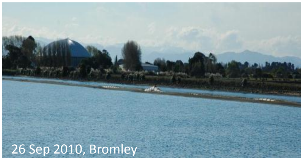
Photo 8.9: Failure of bypass pipelines in the Christchurch WWTP (Source: Author's own)
