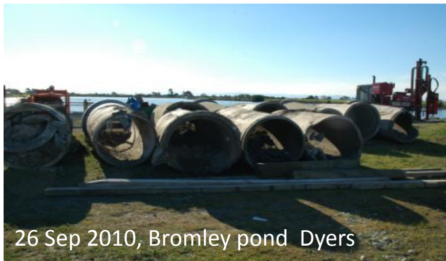
Photo 8.8: Connecting pipe damages in the Bromley pond (Source: Author's own)
