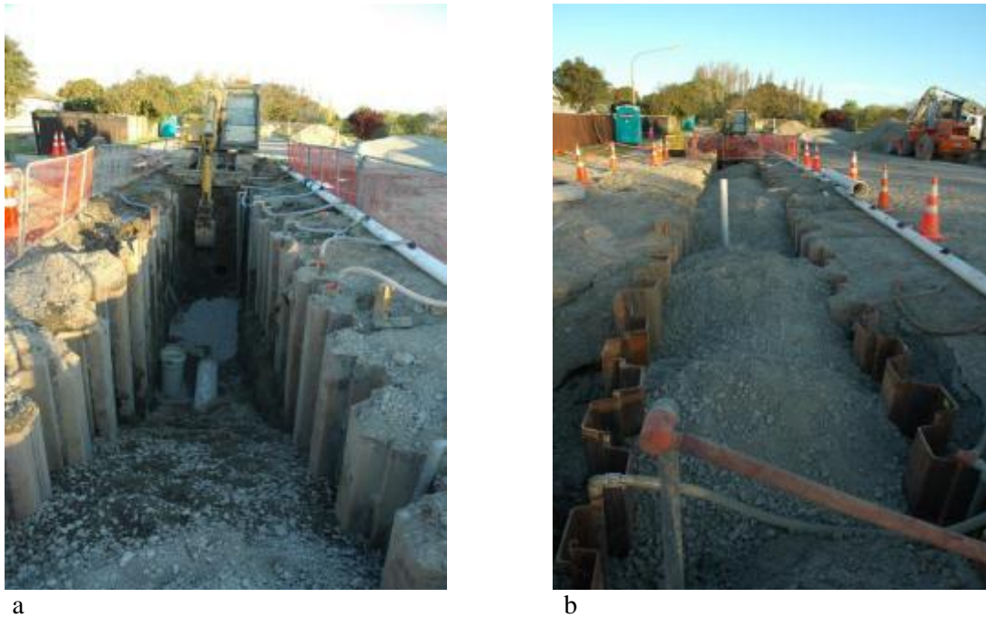
Figure 8.44: Open-cut pipeline replacement in loose sand and high water table (Sep. 2010, Waimakariri district-Kaiapoi) (Source: Author's own)
