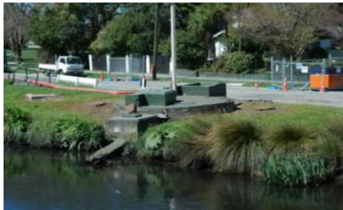
Photo 8.14: WWPS failure due to underground structure replacement (Source: Author's own)
