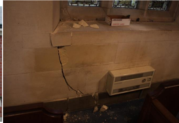
(b) shear damage in the longitudinal walls (mechanism 6), inside (St. Barnaba's, stone, Fendalton)
