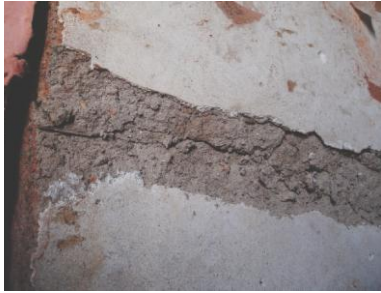
(a) mortar deterioration
