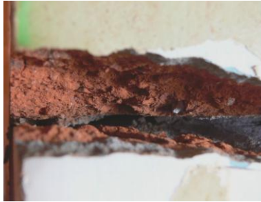
(b) cracking through bricks
