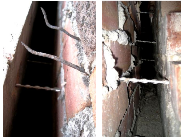
(b) corroded wall ties (left) and newly installed TS ties (right)
