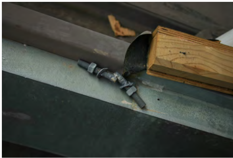
Figure 6-6: Becker, Ross (2011) Eight of these small bolts were all that held up the heavy roof bridging 2 buildings. [photograph] Retrieved on 16 Aug 2013 from Picasa commons: https://picasaweb.google.com/114788127440201076357/2011April27IntoTheChristchurchRedZone?noredirect=1#5602376034129673330 Copyright 2013 BeckerFraserPhotos. Reprinted with permission.
