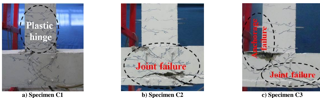
Figure 4. Damage pattern of control specimens C1, C2 and C3 at the end of testing.
