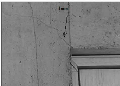
Figure 12 Cracking in the corner.
