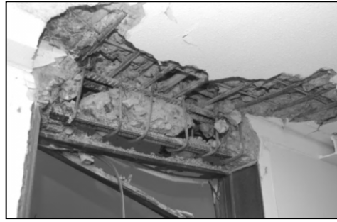
Figure 4 Lack of confinement in lintel
