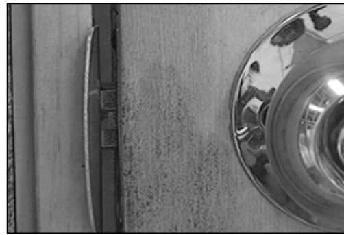
Figure 15 Distortions in the lock.
