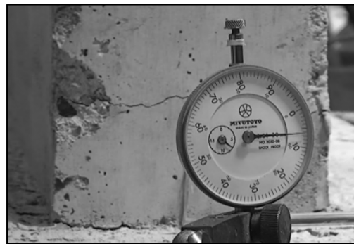
Figure 13 Cracking at the bottom.
