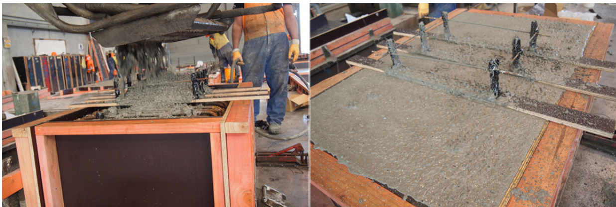
(b) Casting of concrete into foundation block (c) View of the cast-in steel bolt head after pouring
