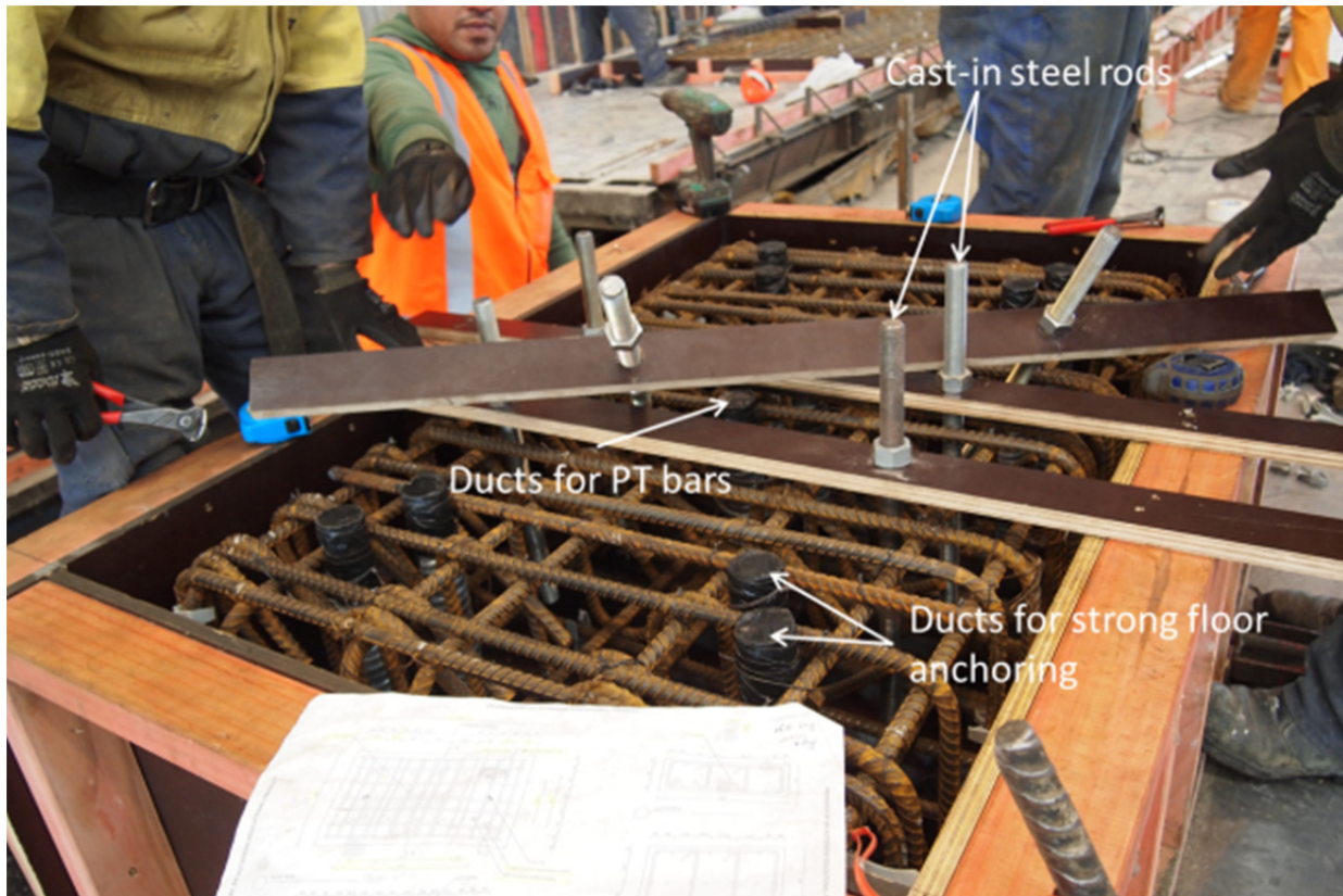
(a) Reinforcement arrangement of the concrete foundation block. Ducts were inserted for tensioning of the PT bars and securing the foundation block to the laboratory strong floor. Cast-in steel rods provided anchorage to the steel base plate
