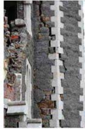
(c) Time Ball Station. Damage to the octagonal tower
