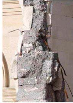
(b) Cathedral of the Blessed Sacrament in Oamaru stone with poured concrete core
