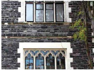
(c) Flexural cracks in the spandrels of Cramner Court.
