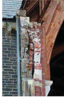
(c) St. Luke's Anglican Church characterized by stone facings with clay brick interior leaves
