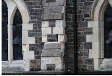
(a) Diagonal cracks in the south façade piers of Christchurch Anglican Cathedral
