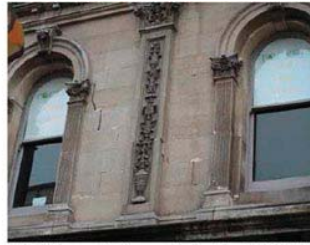
(b) Diagonal pier cracks in the Lichfield Street façade of Strange's Building
