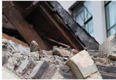
(b) Front façade gable of Former Trinity Church. Presence of original wall-to-diaphragm steel anchors.
