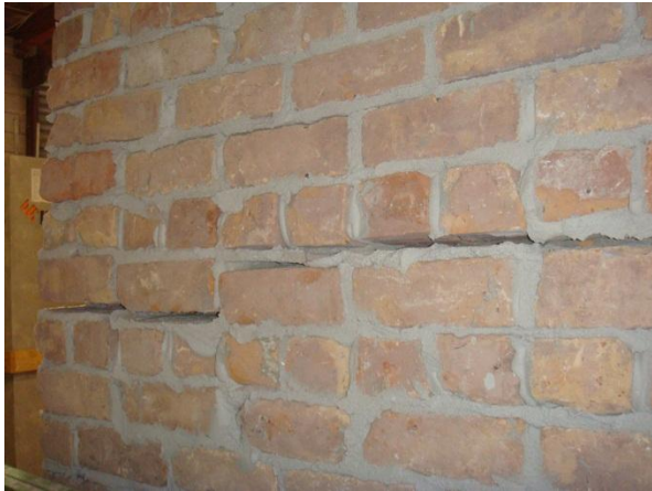
Figure 6: View of the major flexural crack observed on specimen W1-S30-M-CL
