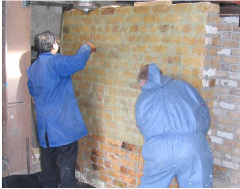
Figure 3: Installation of glass fabric on a wall that was retrofitted similarly to the test wallettes.
