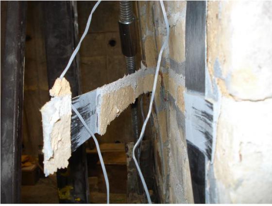
Figure 8: Debonding of CFRP plate.
