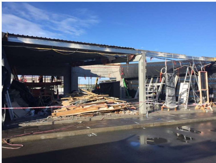
Figure 5.1. Damaged Building in Kaikoura. (Courtesy of Fish and Hunting Kaikoura)
