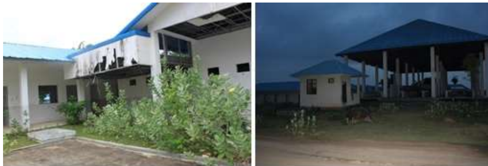
Figure 4.16. Dilapidated and abandoned school and public market place
