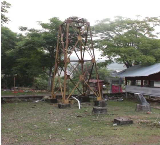
Figure 4.13. Drilled well for drinking water supply
