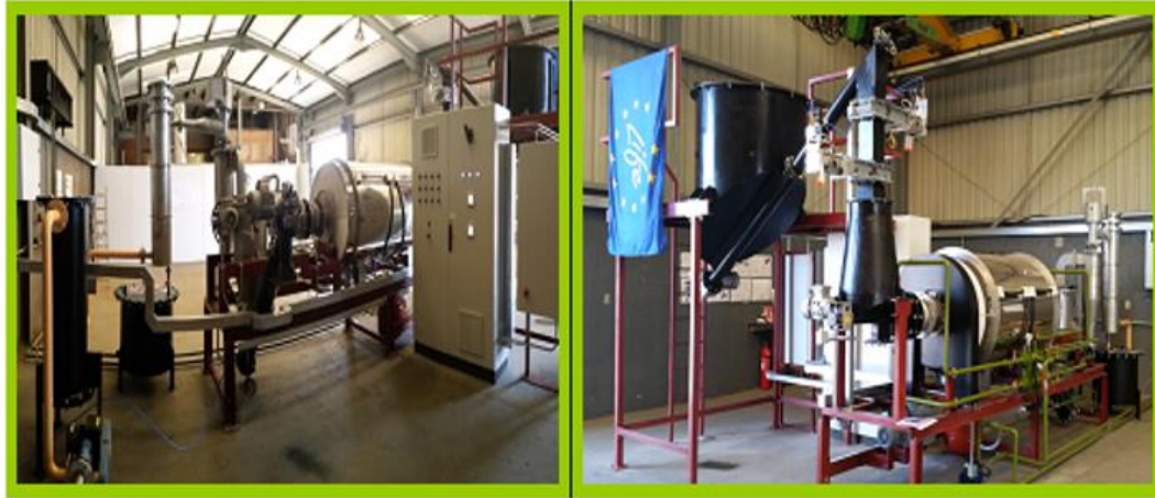
Figure 3. 1. Flow sheet and photos of the pyrolysis prototype (Source: Antoniou & Zabaniotou, 2018)
