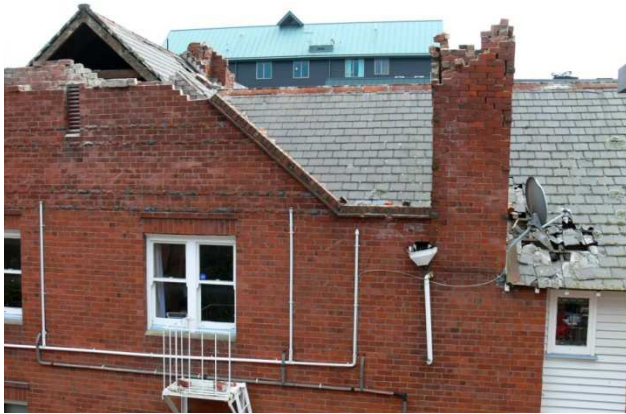
(a) Two damaged chimneys and gable wall.
