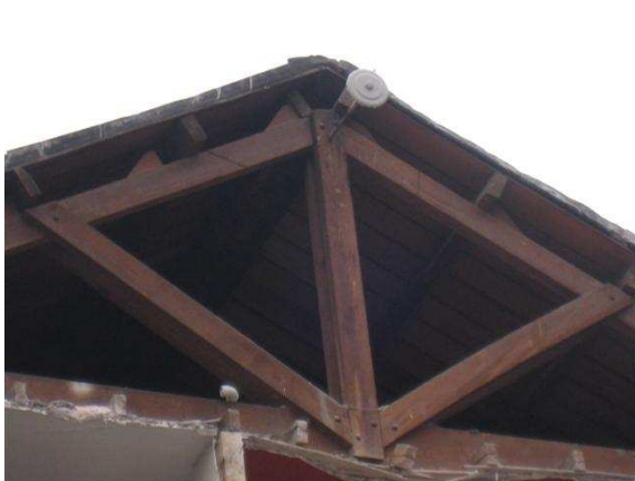
(a) Gable wall failure despite anchor
