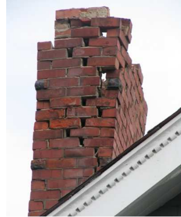
(b) Unstable damaged chimney
