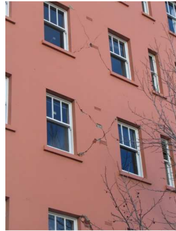
(b) damaged brickwork
