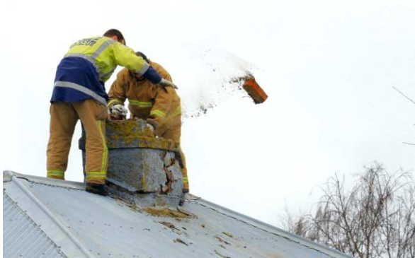
(c) Emergency services remove chimney.
