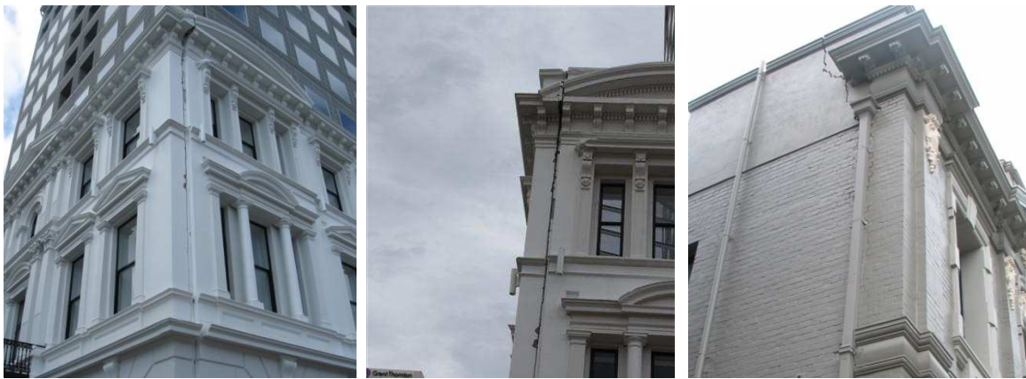
Figure 12. Examples of wall separation at corners of buildings.
