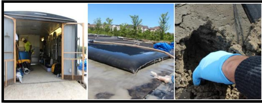
Figure 2-2: Left to Right - Flocculant Pumping System, Geotextile Bags, Sediment after Several Weeks (TRCA & CH2M Ltd, 2016)
