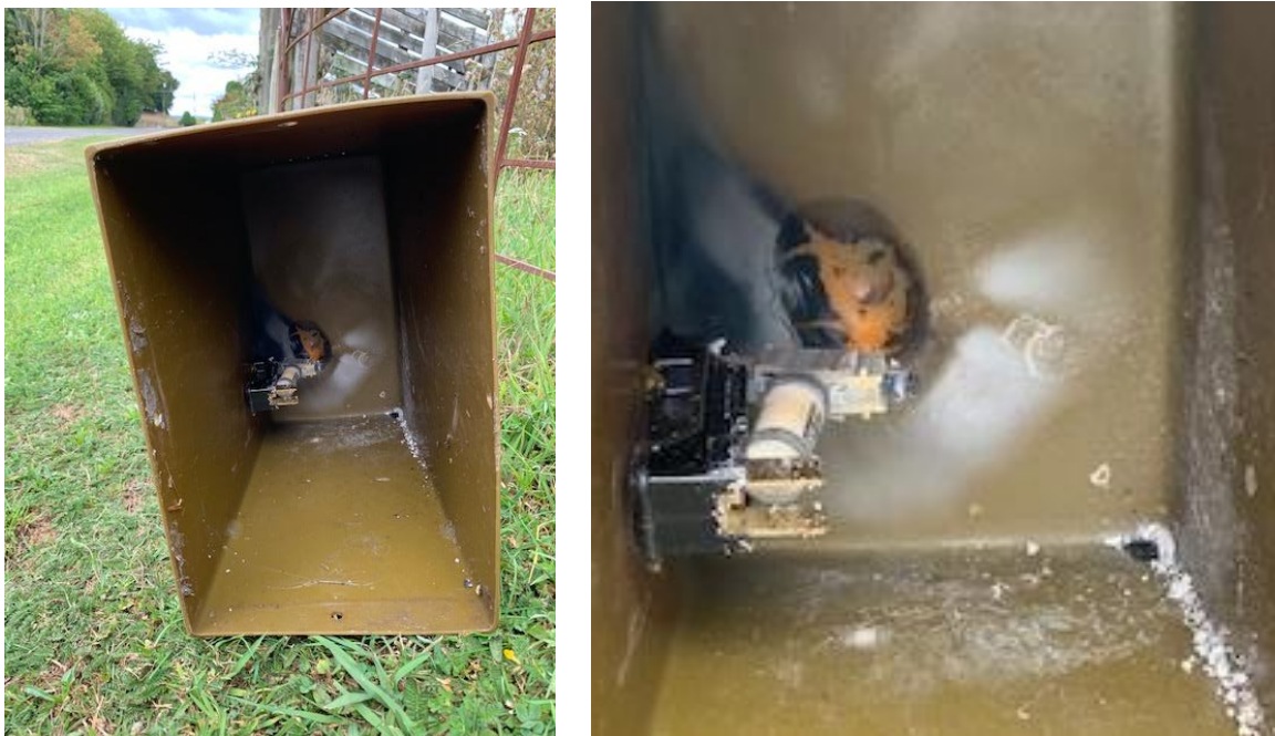
Figure 5 The Fuse Holder Top is Stuck to the PE Pillar Lid and the Lid Shows Signs of Sooting and Melting. The Mounting Plate Shows that the Plastic Has Melted and Dripped Away Behind the Hot Connector.
